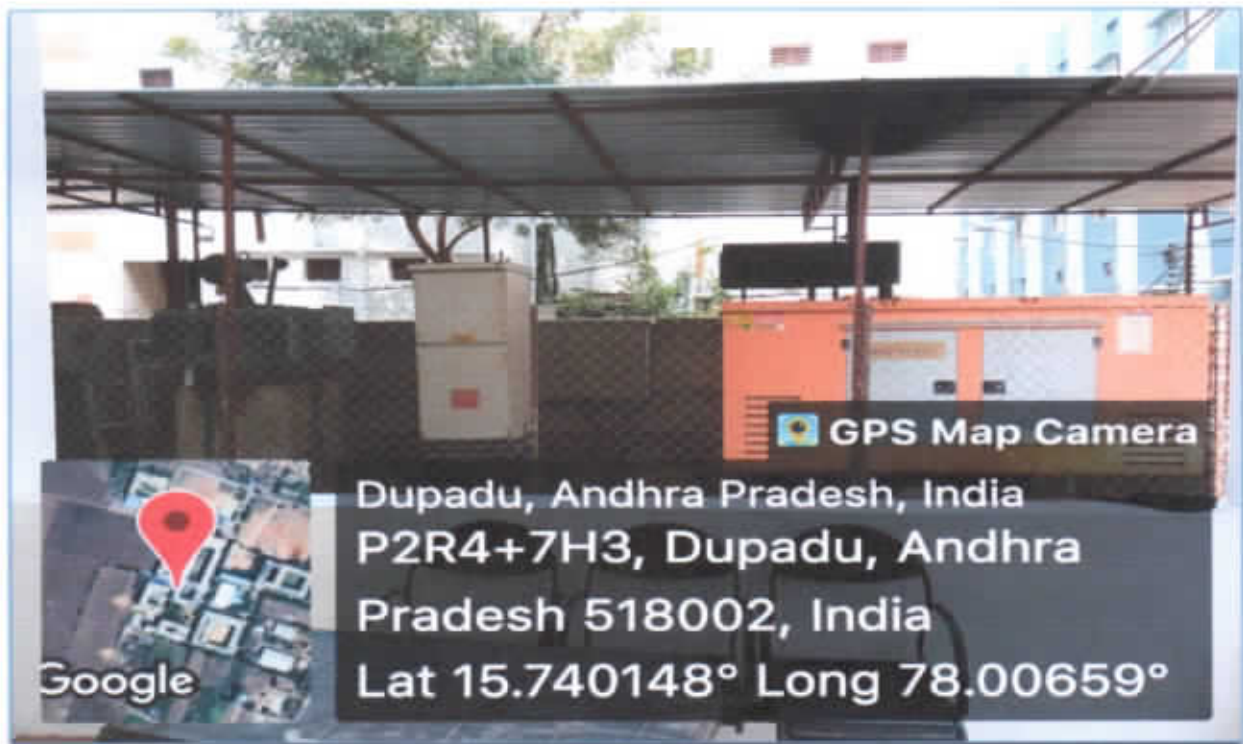
Fig. 7.1.2.3 generator to the Dr. KVSP
